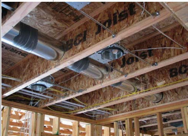
Running ductwork and trunk lines through the web brings the entire system into conditioned airspace.
